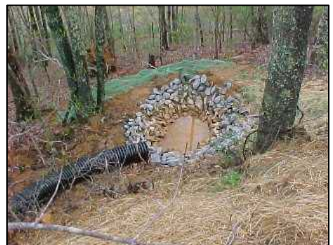
Check dams made from mulch socks (top) and temporary sediment traps (bottom) are two structural barriers to sediment movement.
