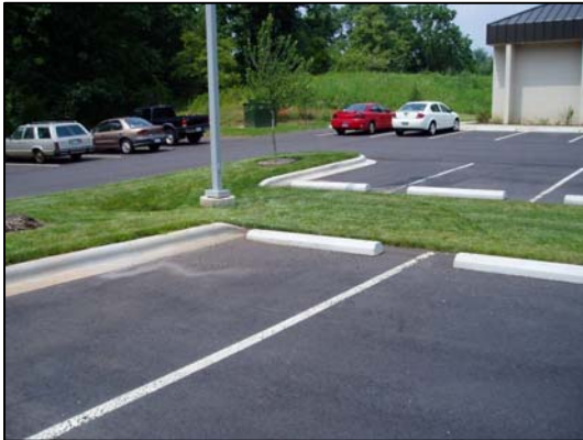
Bioretention areas like the one shown above are one type of vegetated swale.
